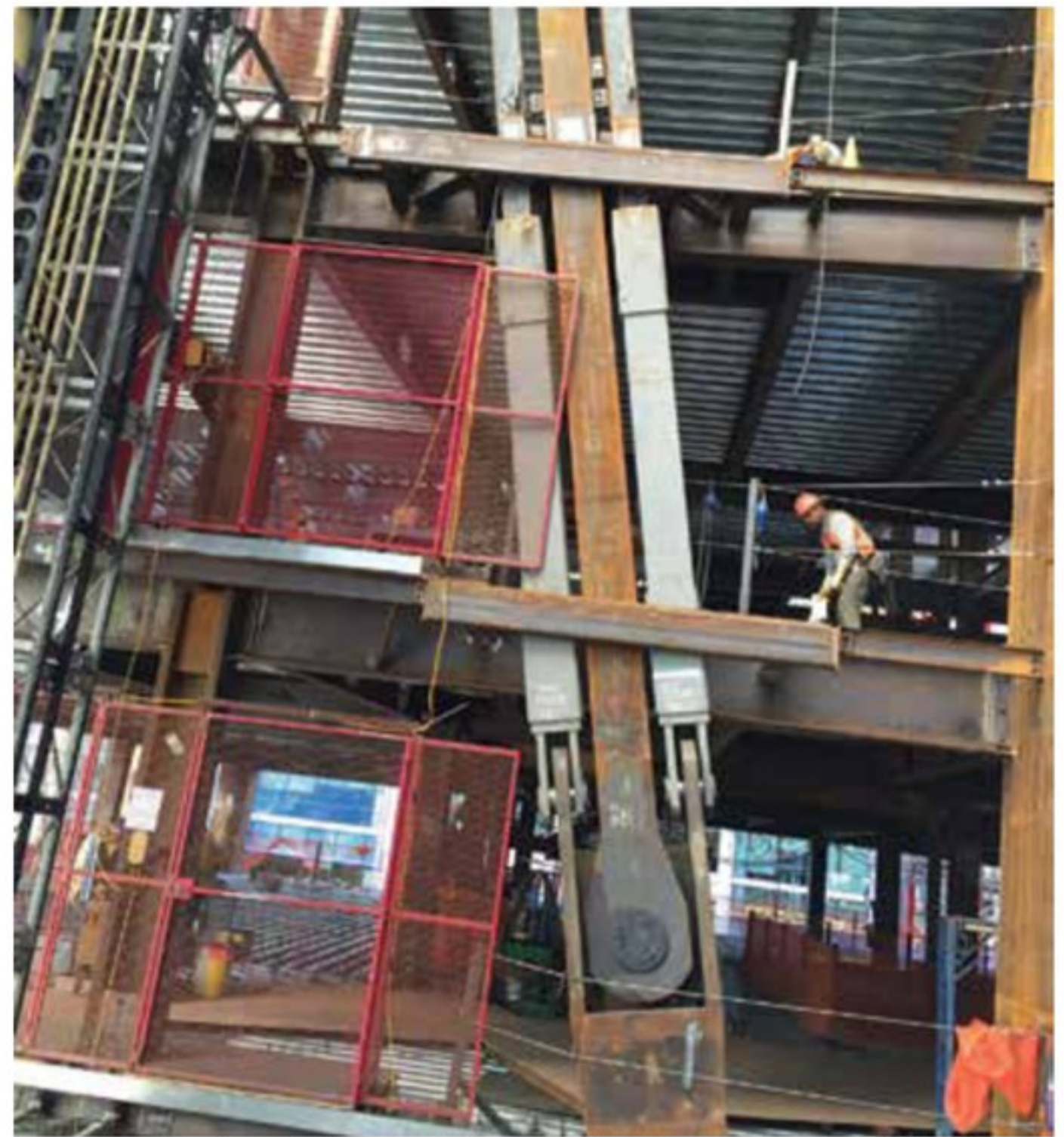
Figure 7. At each end of the mega-brace, the connections are pinned. At the lower end (shown), BRBs are introduced into the load path of the secondary braces.
